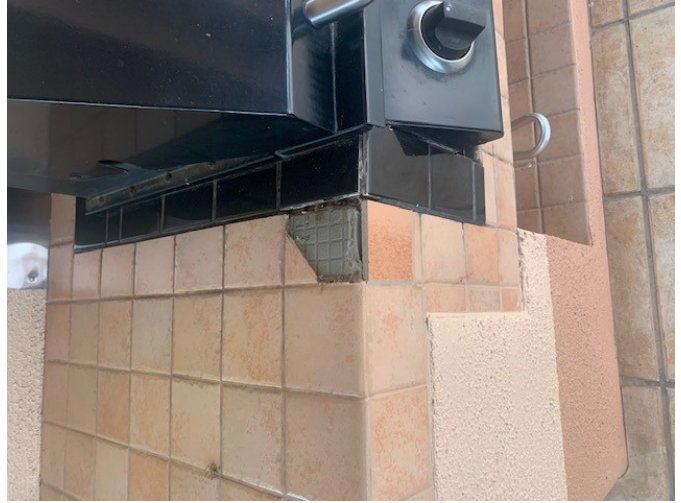
Tile missing at countertop.
