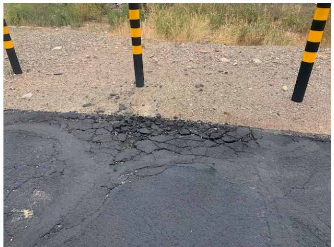
Isolated areas of deteriorated pavement.
