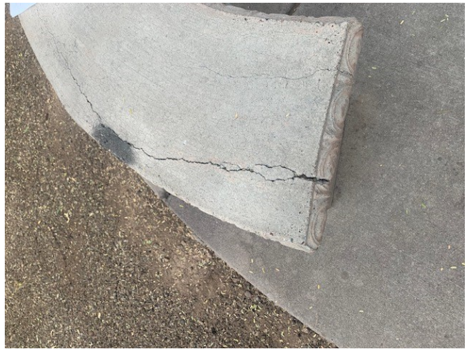
Concrete bench deterioration/crack observed.
