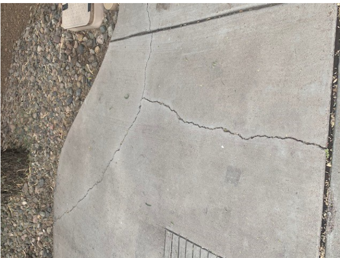
Isolated pavement cracks.
